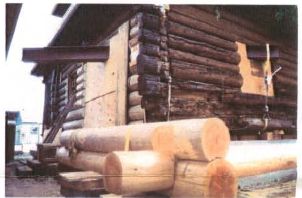
1996/7 preservation of the Log House Museum, showing the damaged south wall, with the new replacement wall being created alongside. (Courtesy Deborah Mendenhall, SWSHS Collection)
